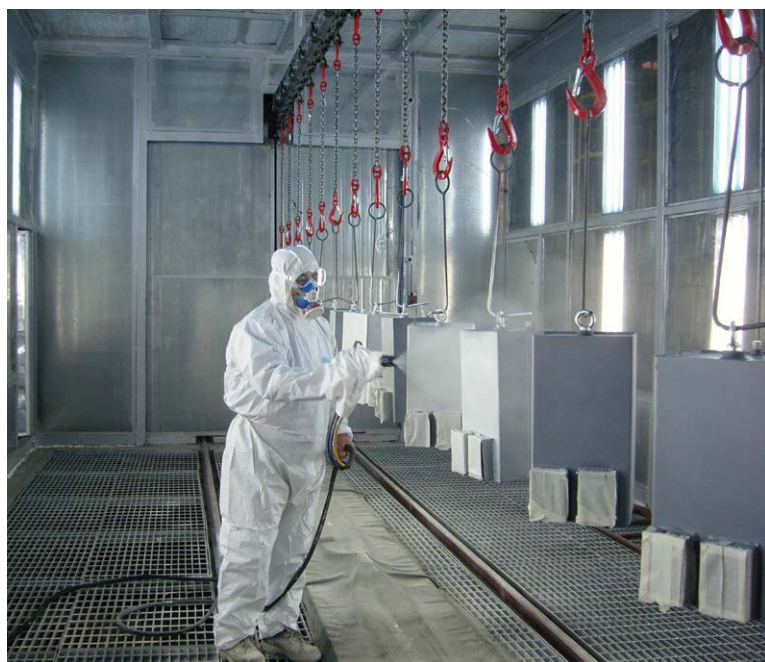
An automated painting line has been installed.
